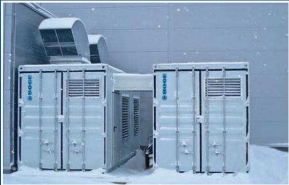
Container station for extreme environmental conditions.
